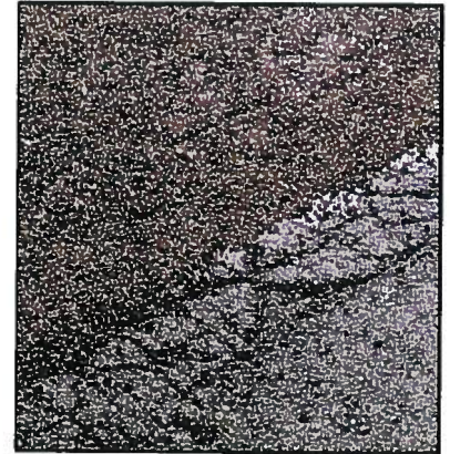
A thin application of LWA shows oil around the particles next to the exposed edge of the old deteriorated road surface.
