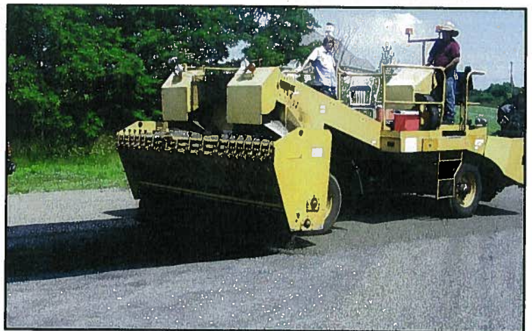
ASTM #9 LWA applied at 130 SY/CY over RS-1P Emulsion at 0.20 to 0.25 GAL/SY in a rural, residential cul-de-sac in Buchanan County, MO
